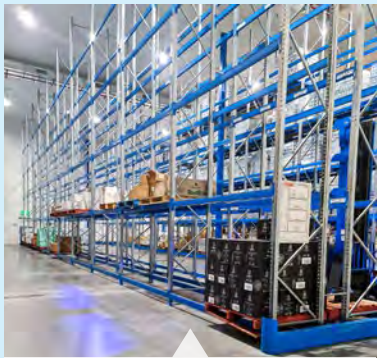
Larapinta Cool Room
