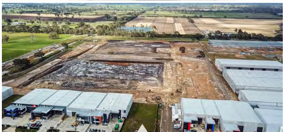
Earthworks at Dandenong South – You can see the outline of our buildings!
